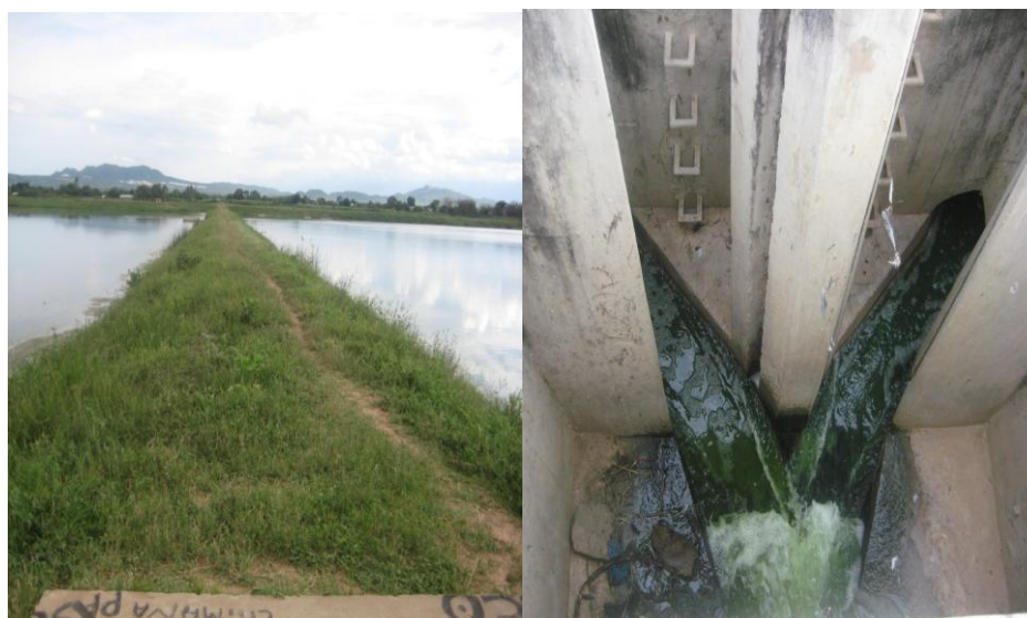
Figure 3. Swaswa wastewater stabilization pond in Ipagala Ward in 2013.
